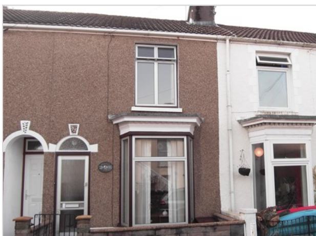
Changes to wall finishes, door and window openings and frames remove the heritage character and the rhythm of the terrace
